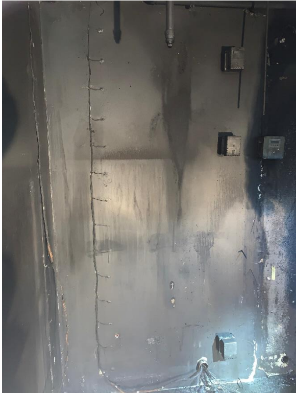
Figure 145 – Condition of side wall next to the Initiating Unit after Test 3.
