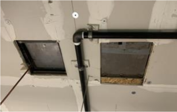
Figure 13 – Positive pressure relief vent (left) and negative pressure relief vent (right).
