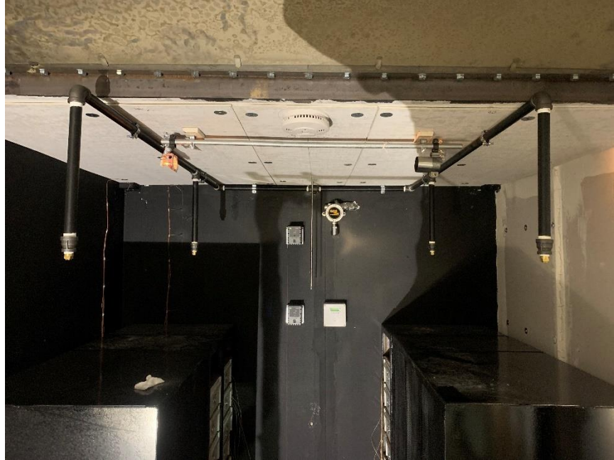
Figure 16 – Location of four water suppression nozzles above ESS unit enclosures.
