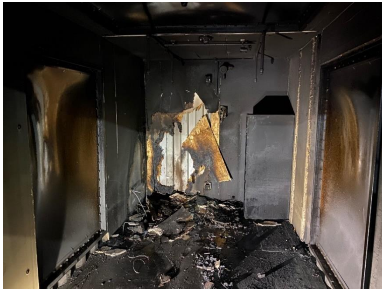
Figure 39 – Thermal damage to walls photographed during test termination and overhaul after Test 1.
