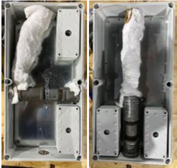
Figure 29 – Heat flux gauges installed for Left Target Unit (left) and Front Target Unit (right),
